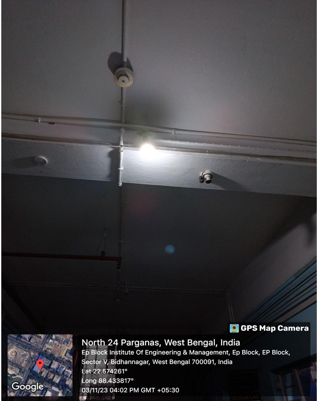
Photo: LED Bulb in Corridor
