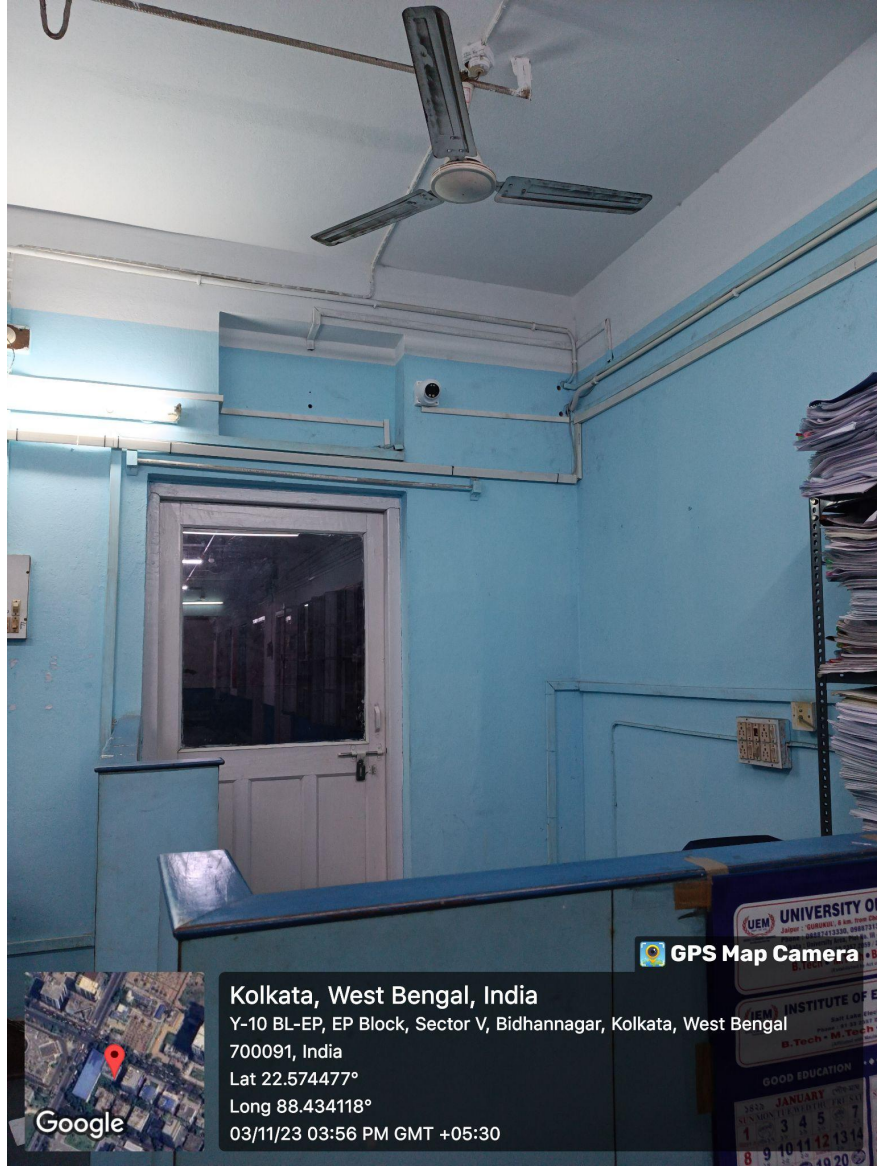
CCTV in all the faculty rooms
